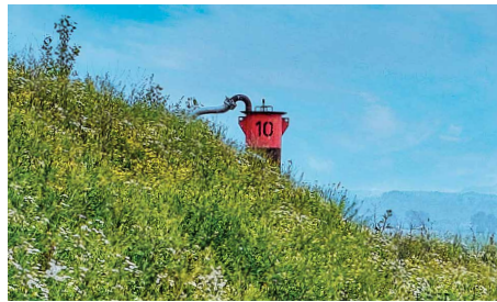
Gasbrunnen Zentraldeponie Cröbern (Foto: ZAW)
